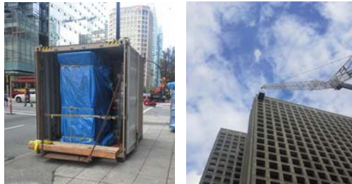
1075 West Georgia Project: Equipment ready to be unloaded, and later being flown up to the 27th floor by a 475 foot crane.
