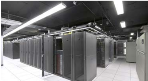
Cologix's 15,000 square foot data centre at 1050 West Pender was built to meet pent up demand and create a more efficient on-ramp to global networks and clouds.
