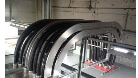
1075 West Georgia Project: Single conductor cables from the secondary side of one of the transformers to the 600V distribution.
