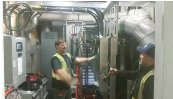
West Vancouver Transit Center Generator project, Joel Logan and Leonard Deza completing final terminations.
