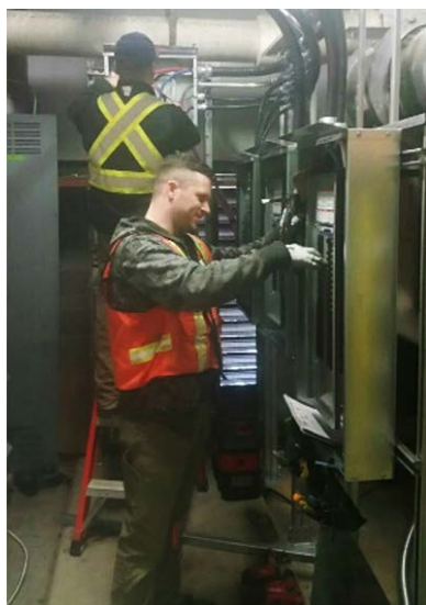
West Vancouver Transit Center Generator project, Chad McCormick and Leonard Deza making space where they can for new ATS & panels.
