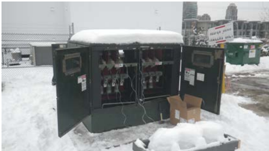
Despite rain, sleet or even a few inches of snow, the crew at Southgate still managed to complete all the HV terminations without a hitch.
