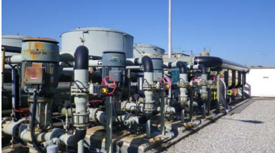
Keeping the fuel flowing making sure all eight out-bound pumps are in good working order at YVR.
