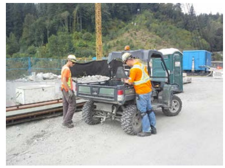
Nathan Townsend left and Brad Solven prepare for another day's work at the Ruskin dam. The project will take an estimated 30 more months.
