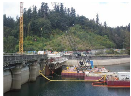
Temporary dam bulkhead with 275 tonne barge crane located on the upstream side of the dam for removal of existing gates. Operational gates at left of photo.
