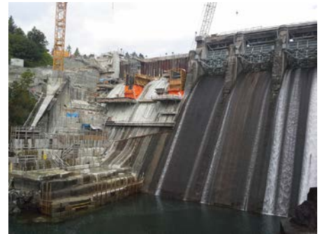
Looking across the Stave River. Old gates 1,2,3 have been removed. New pier 2 & 3 formwork started. During the upgrade project the dam continues to generate power to the lower mainland.
