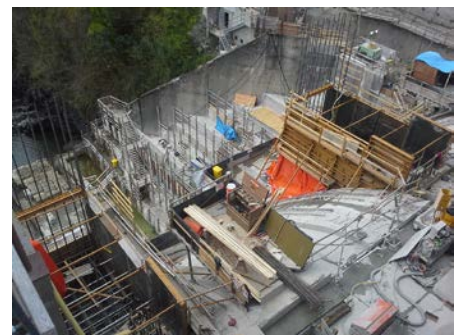
Looking down into the new pier gate formwork. A new gate control building will be constructed at the top of each pier in addition to the main control building on the east side and a backup control building on the west side.
