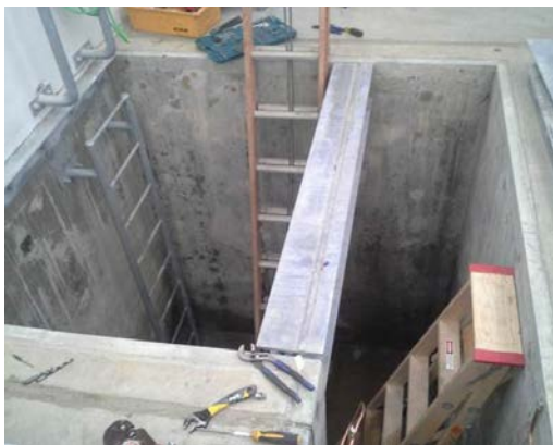
Electrical Pit in a Receiving Station
