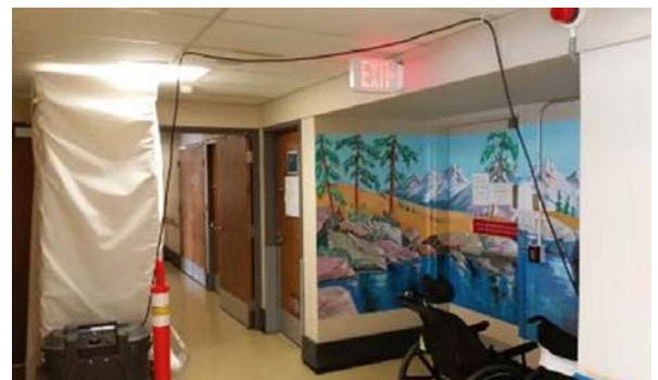
Extension Cord Suspended with T-bar Clips
